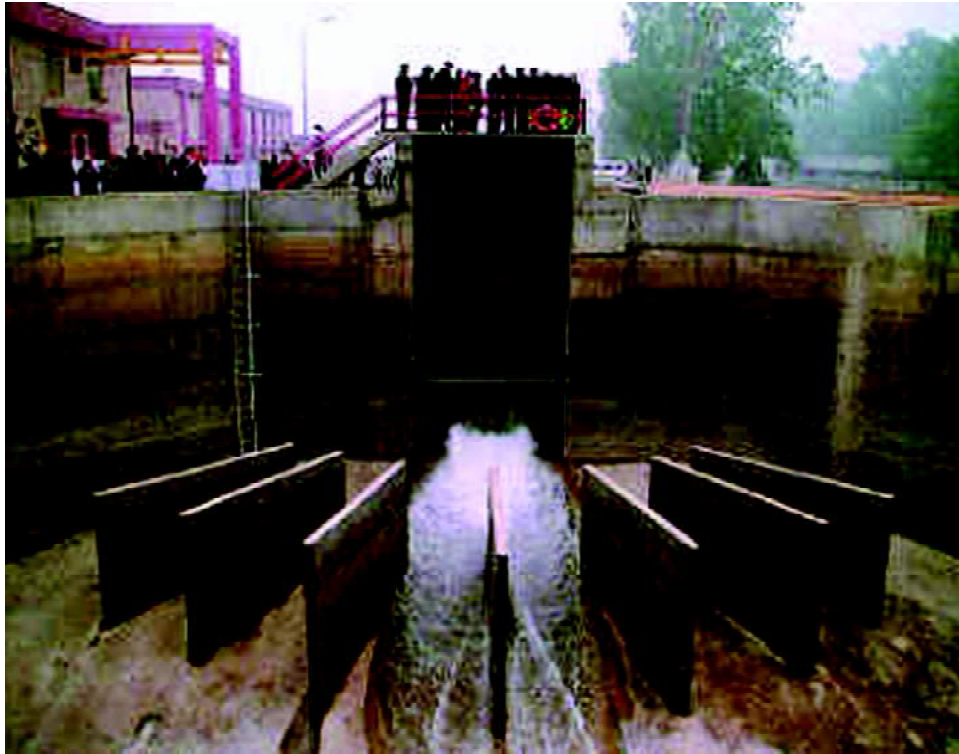
Fig. 18.10 : Water treatment plant
