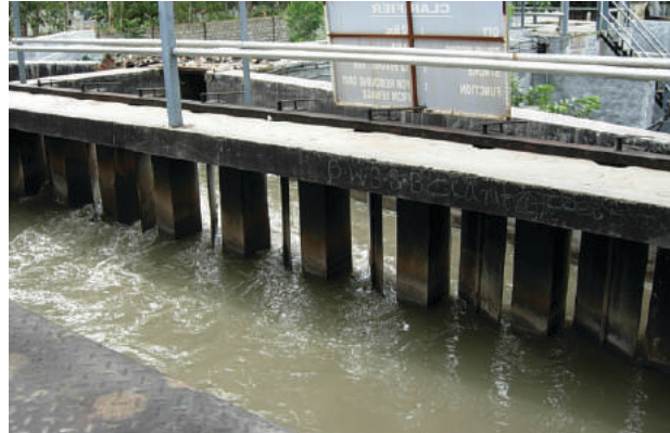
Fig. 18.4 Grit and sand removal tank
