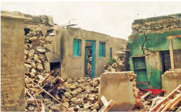
4.2 : Effects of the earthquake at Killari
