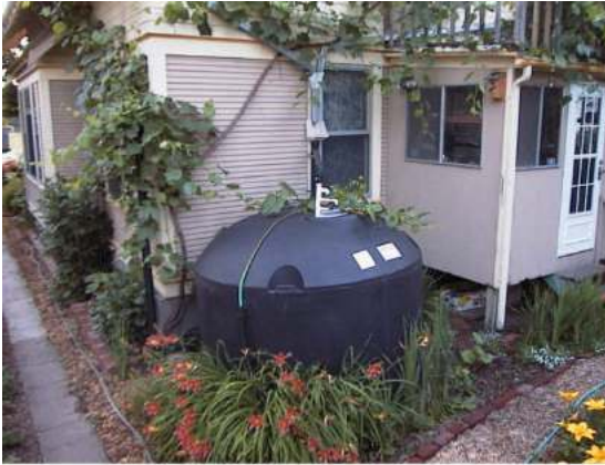
Rain water storage tank
