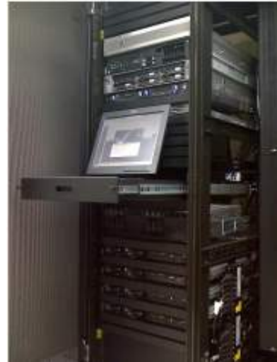
Fig. 4.5 : Rack mounted servers
