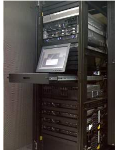
Fig. 4.5 : Rack mounted servers
