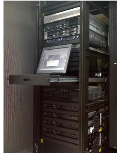
Fig. 4.5 : Rack mounted servers
