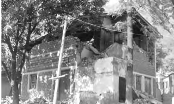
Figure 7.1 : A Damaged Building Due to an Earthquake
