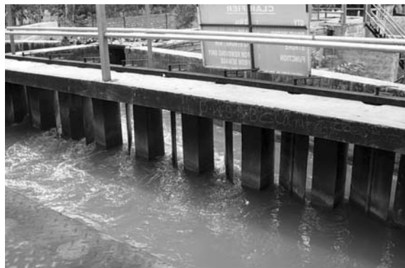
Fig. 18.4 Grit and sand removal tank
